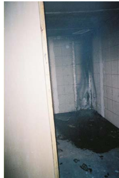
Fig. 7 Fire damage to panels
